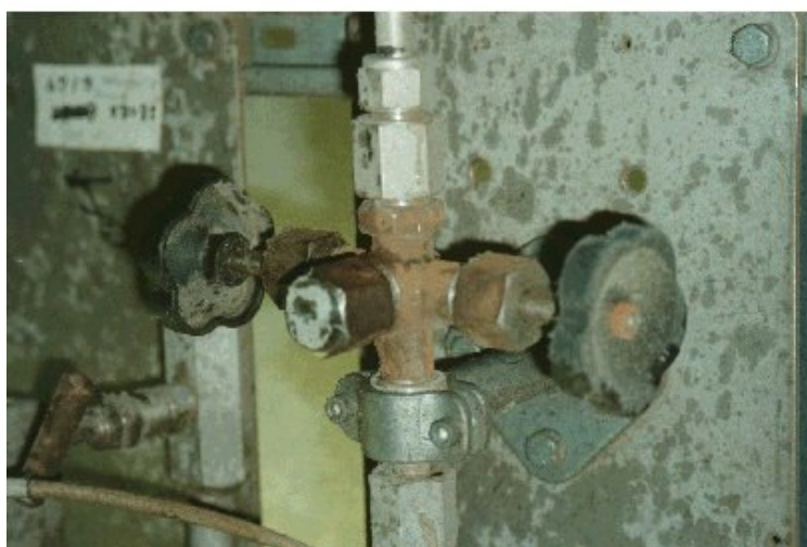
Figure 17 Corroded aluminium isolation plates and steel valves.
